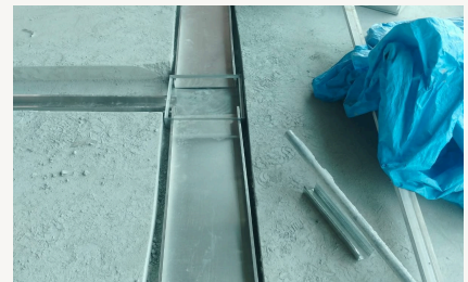
Floor track and service run
